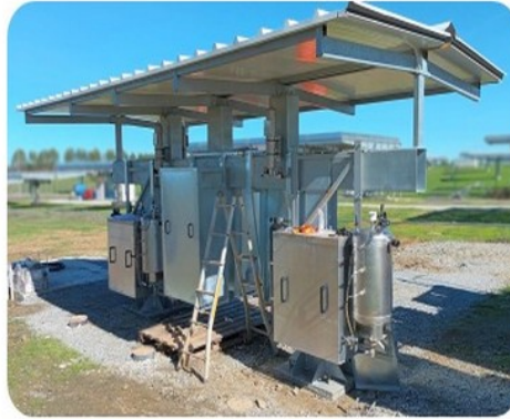
HEVO-Chain demonstrator installed in Évora
